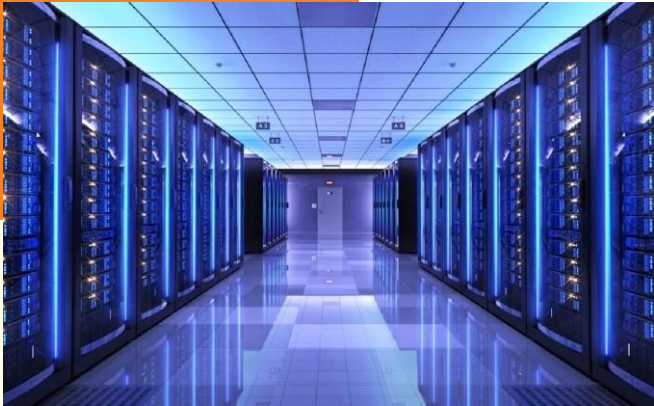
Data Centre - Hyderabad
