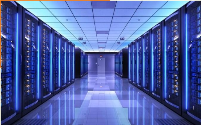
Data Centre - Hyderabad
