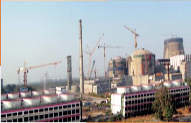
Kakrapar Atomic Power Project High Volume Fly Ash in Nuclear Reactor Dome Construction -Gujarat
